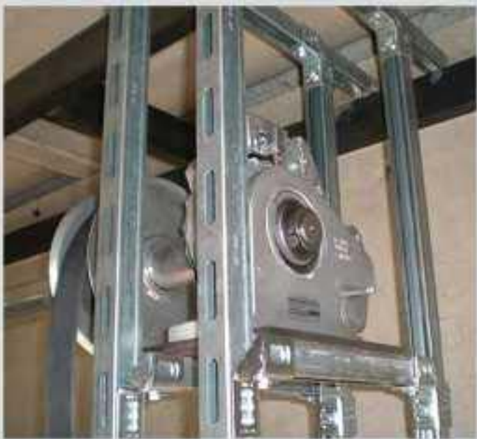
Detail of the anti drop device and main structure with HILTI profiles
